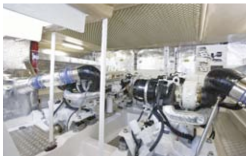
The C12 715hp Caterpillars proved to be economical, while also delivering good performance.
